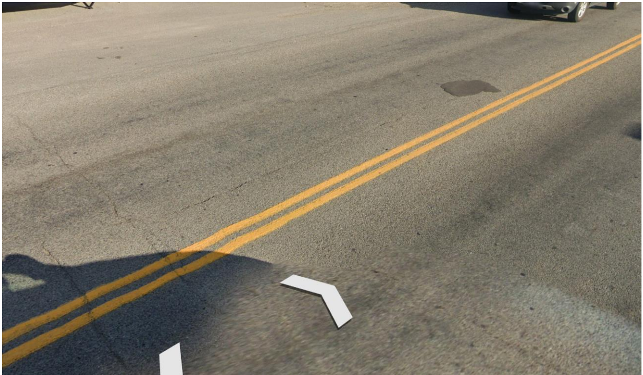
Woodruff pavement cracking, rutting and potholing.
