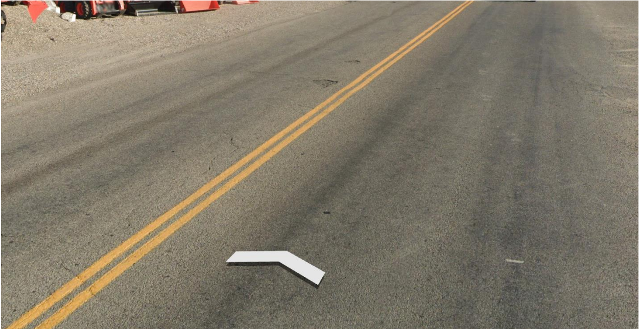
Woodruff Pavement Conditions (cracking and potholing)
