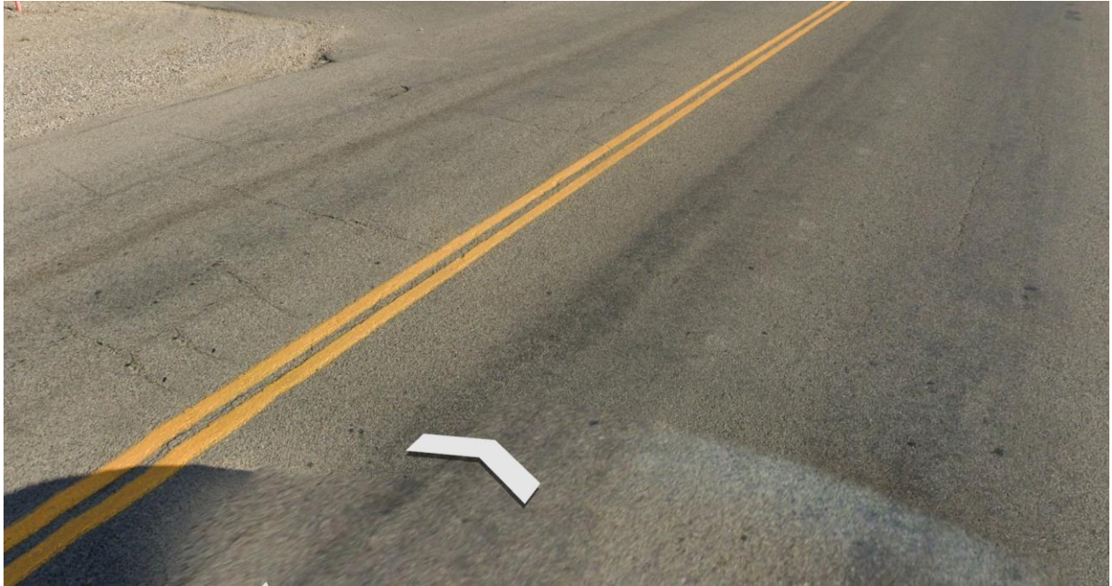
Woodruff pavement cracking and rutting
