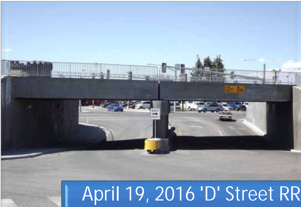
September 16, 2009 'D' Street RR Underpass deterioration
